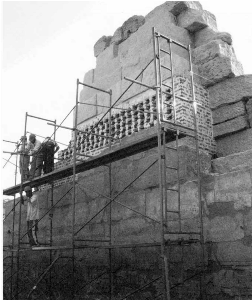
Brick buttress with upper vener blocks in place, from the south. Dany, Mustafa, Saber, and Sayid (below).
